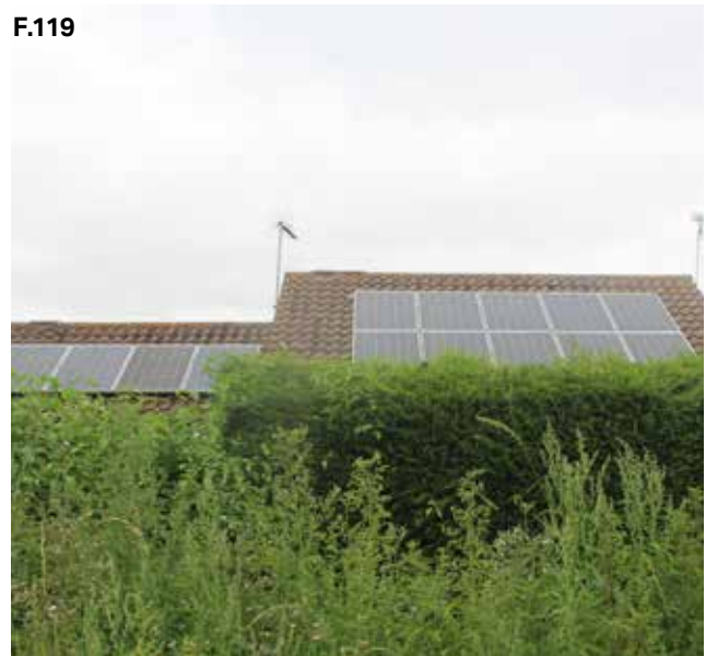
Figure 119: Solar panels installed on the south-facing pane of the roof of new build house in Wetheringsett
