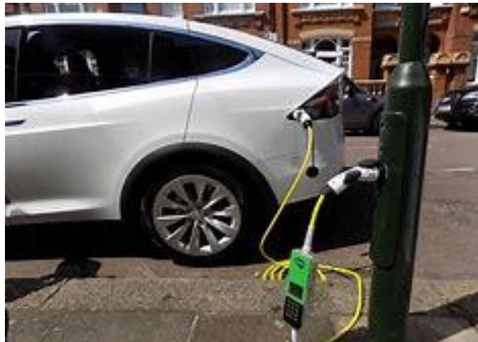
Figure 1: Light column-fitted electric vehicle charge points 7
