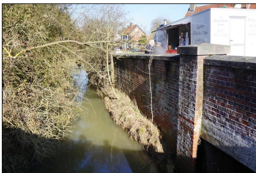
Figure 3-3: Aspoll Road culvert skew at Market Square
