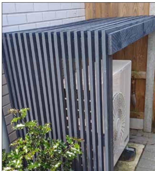
Figure 56: Example of a discreet air source heat pump cover.
