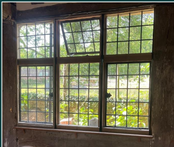
The same window from inside – The secondary glazing has been removed from the central and right-hand side casements. The secondary glazing on the left-hand side is barely noticeable
