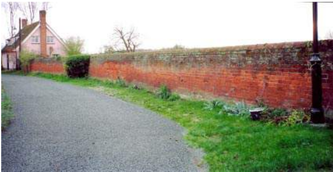
Red brick wall for 41 metres, approximately, between No. 1 and No. 15. Possibly contemporary with the building of No. 1.
