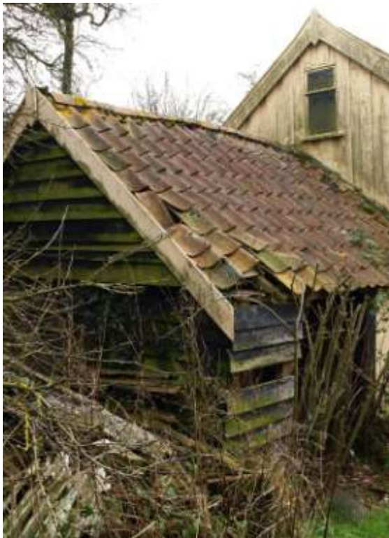
In Need of Repair
